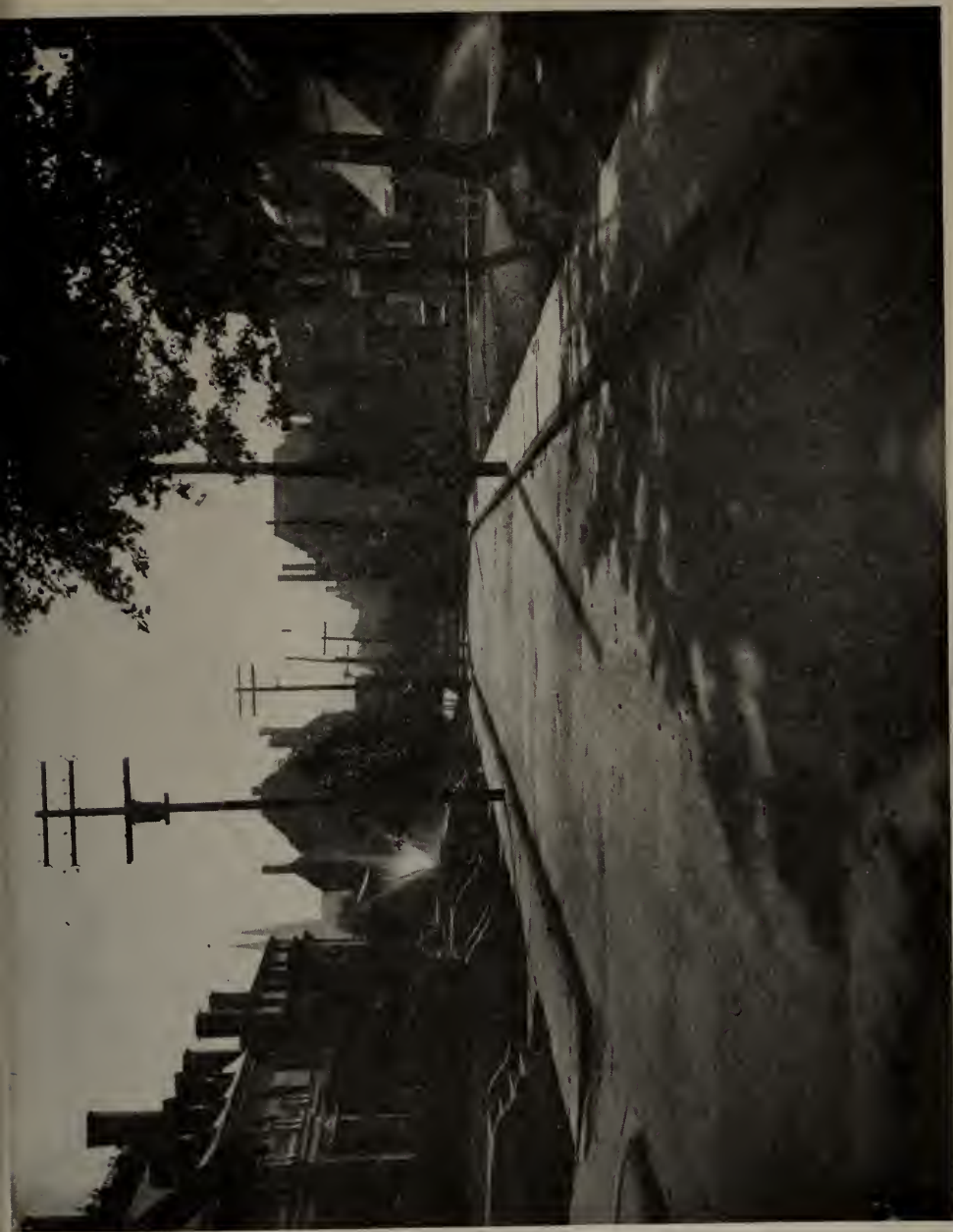
Showing the patched condition of Castleman Street, only about \frac{1}{4} of the original surface left—showing
